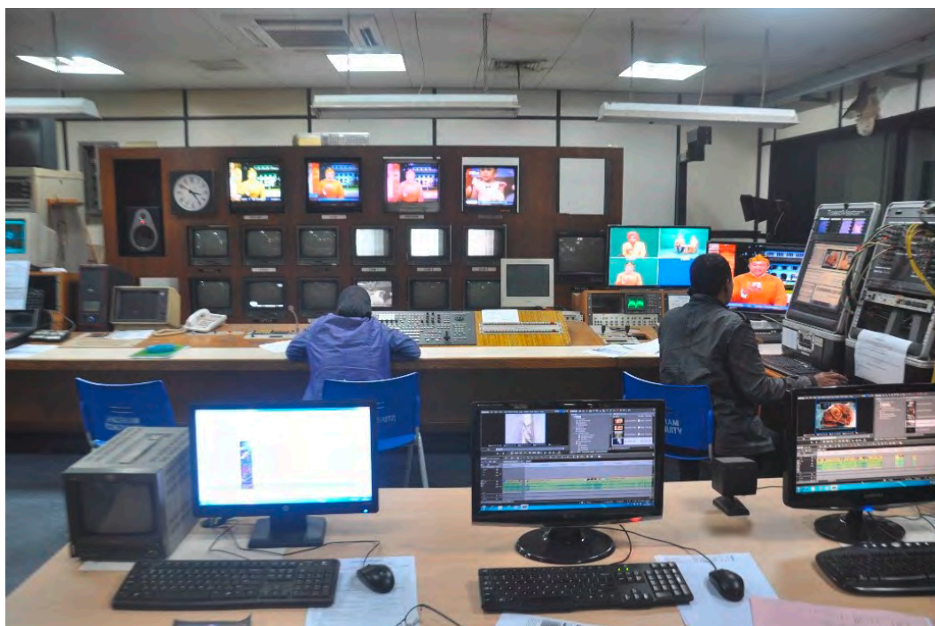
Gambar 1. Master Control Room TVRI LPP Jawa Barat
